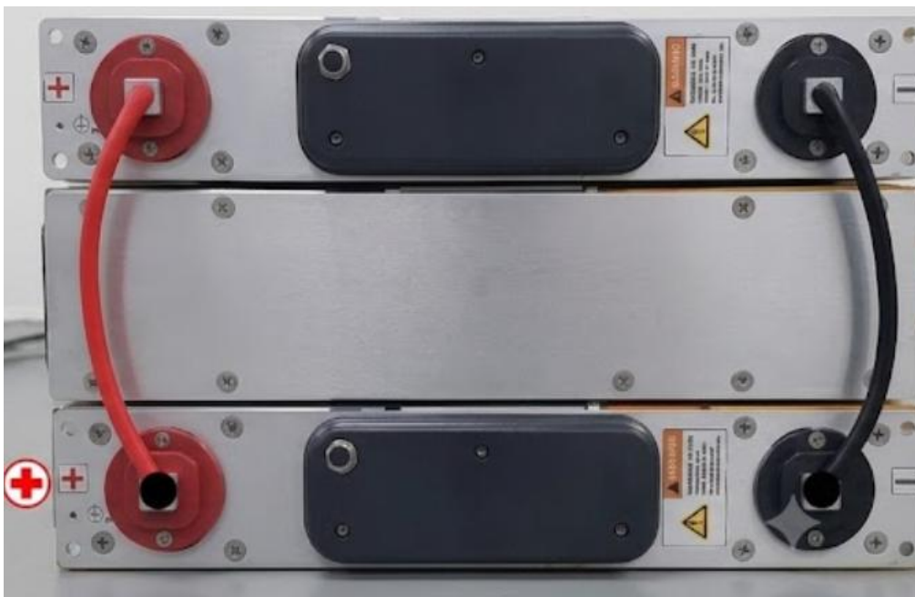
Figure 5: Parallel connection of PBLH-54R0/166SDHV modules
